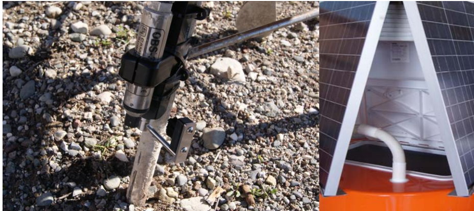
Figure 4. Pictures of turbidity optical sensor and humidity sensor located on a floating buoy deployed in Asprokremmos Dam
