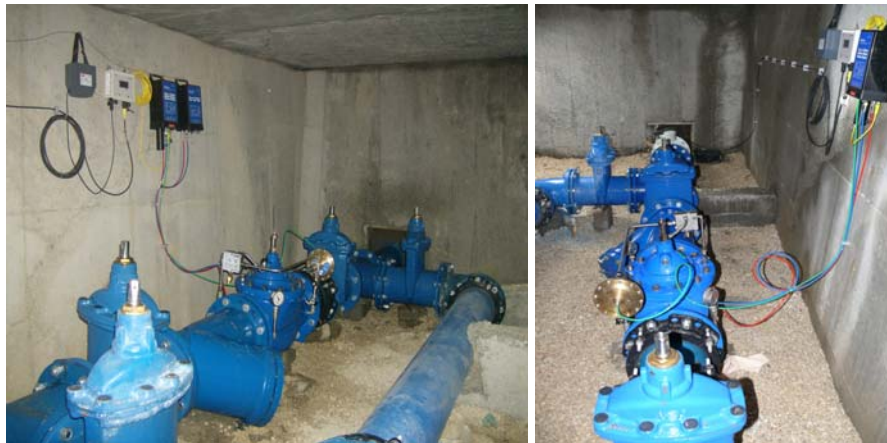
Figure 2. Flow meter and PRV chamber
